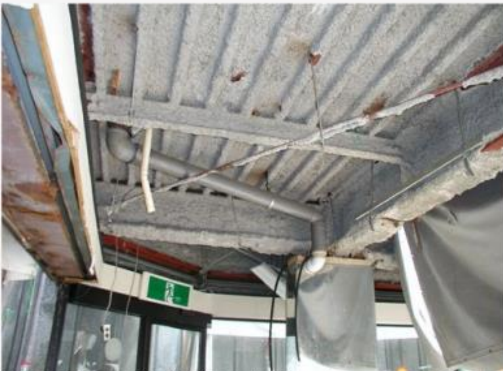
Renovation of ceiling. Asbestos was exposed.
